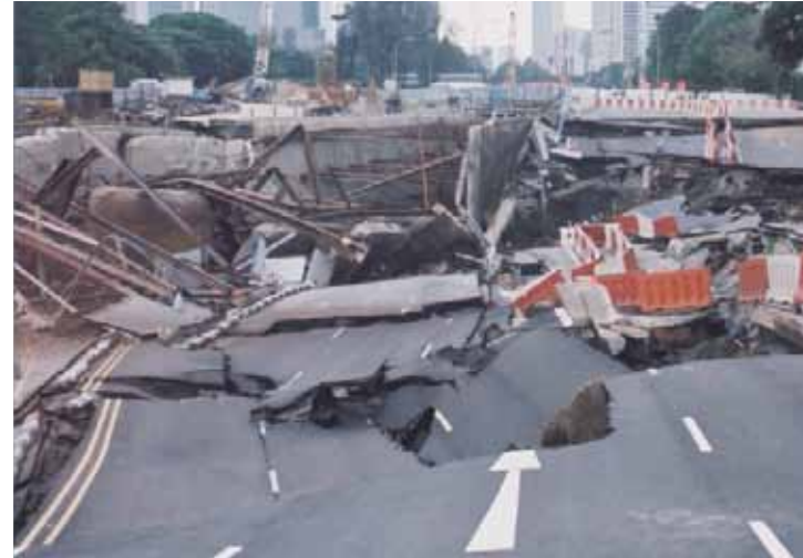
Picture (top left): A section of the Nicoll Highway that caved in.
