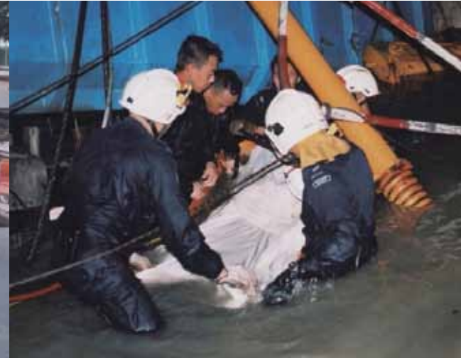
Picture (top centre): DART rescuers extricating one of the four missing workers from a partially submerged cavity.
